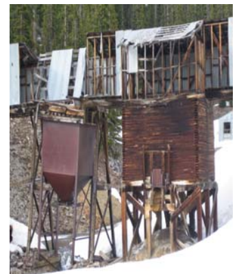
Above: Removing the trestle and ore bins were a small part of the overall cleanup at the Standard Mine site. Courtesy of the EPA.
